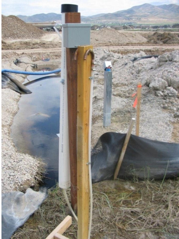
Figure 3-5. Manometer Settlement Platform
